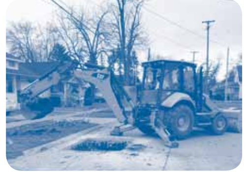
Service line replacement work required by the State's Lead and Copper Rule
